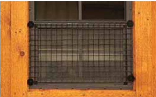
Wire over window
